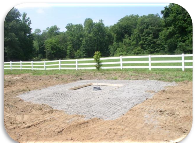
This livestock waterer, under construction for horses, will eliminate the need for access to creeks and streams and reduce manure discharge into our water supply.
