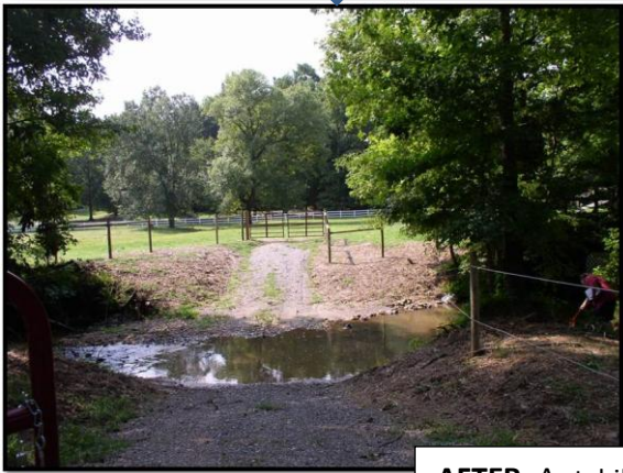
AFTER: A stabilized livestock stream crossing protecting water quality in Falls Lake
